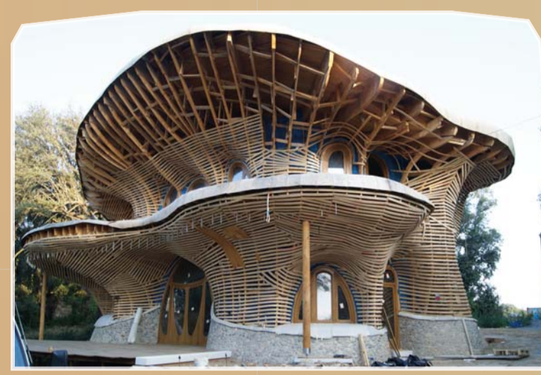
Construction of an organic building made of wood, stone and clay from the site. El Palol, Spain. arc.cz/to/organicbuilding
